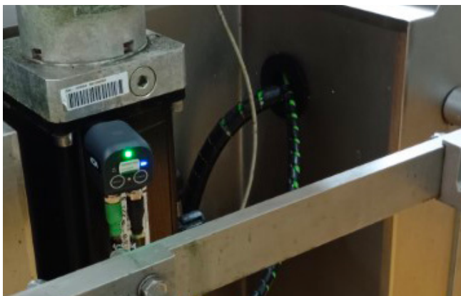
SmartCheck installed on servo motor.
