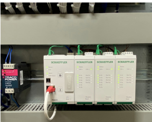
Schaeffler ProLink CMS in switch cabinet.
