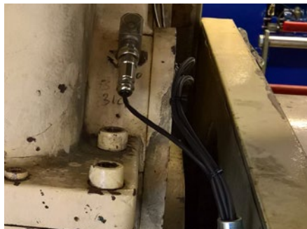
Internal and external sensors of the gearbox
