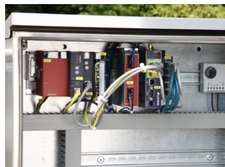
Switch cabinet : MELSEC System Q and eWon Router
