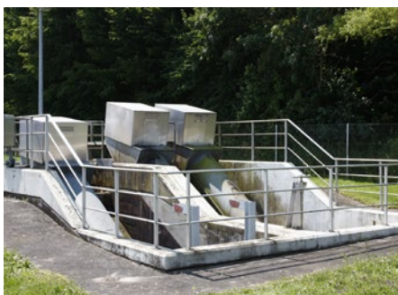
Return activated sludge pumping station
