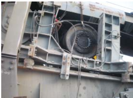
Shaft failure on tension/take-up pulley
