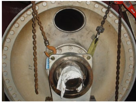
Slings and chain blocks around the dryer
