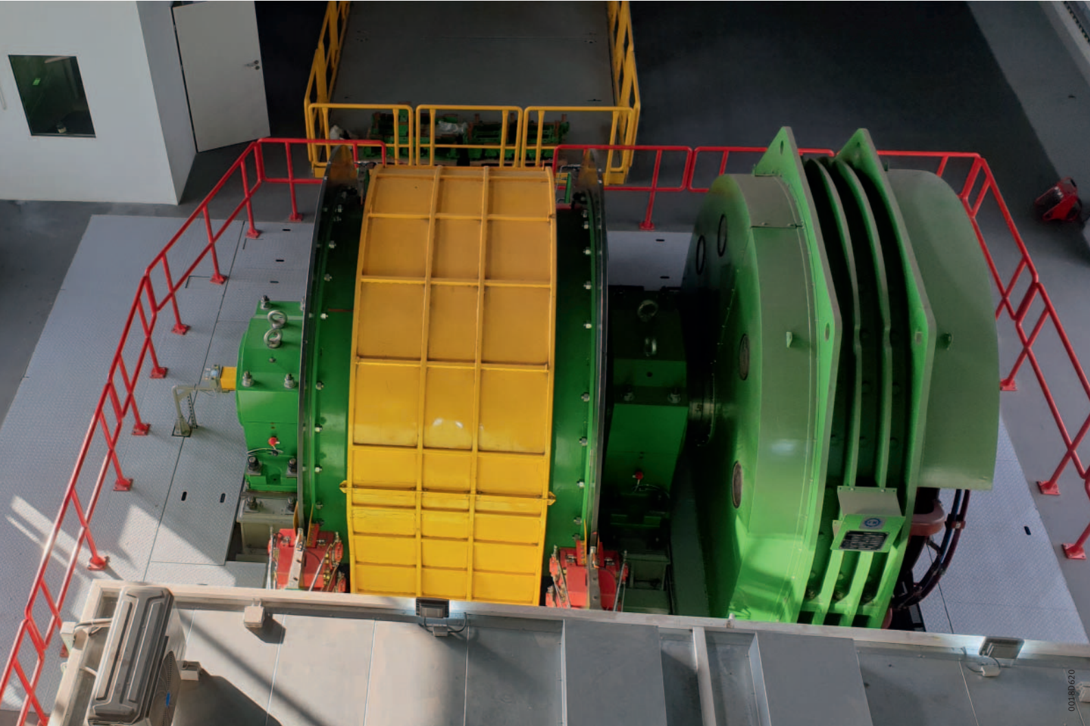
View of the heart of the copper mine shaft L-VI in Lubin – the hoisting machine from MWM Elektro
