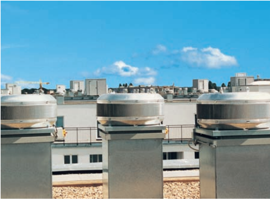
Roof fans (Photograph courtesy of TLT-Turbo, Bad Hersfeld)
