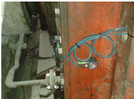
Two FAG SmartCheck units monitored temporarily the condition of the trunnion drive end bearing
