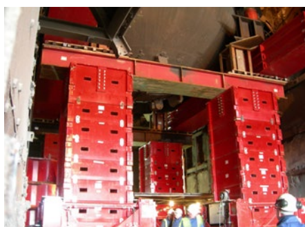
Supporting structure for vessel
