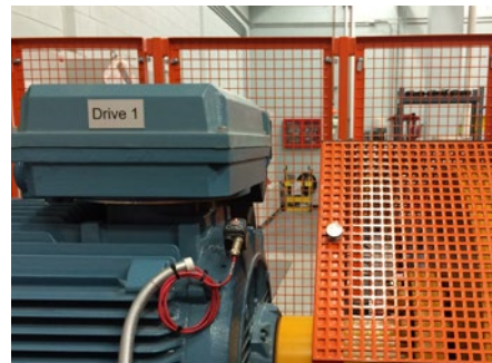
Monitoring of motor vibrations using the FAG SmartCheck
