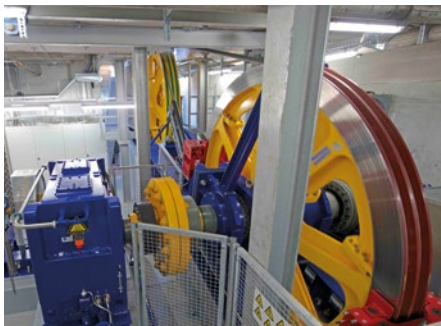
Drive train in one of the two mountain stations
