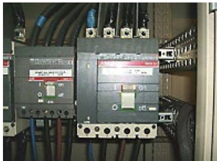
Low voltage cabinet
