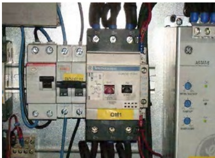
Low voltage cabinet
